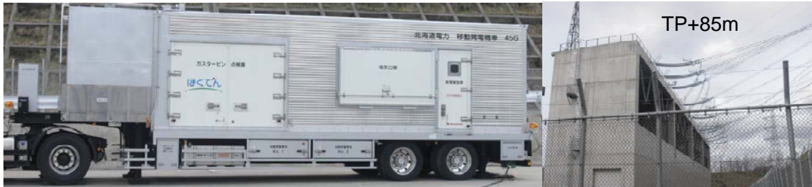
(a) 4000 kVA mobile gas-turbine generator at 31 m parking and GIS at 85 m height (Hepco).
